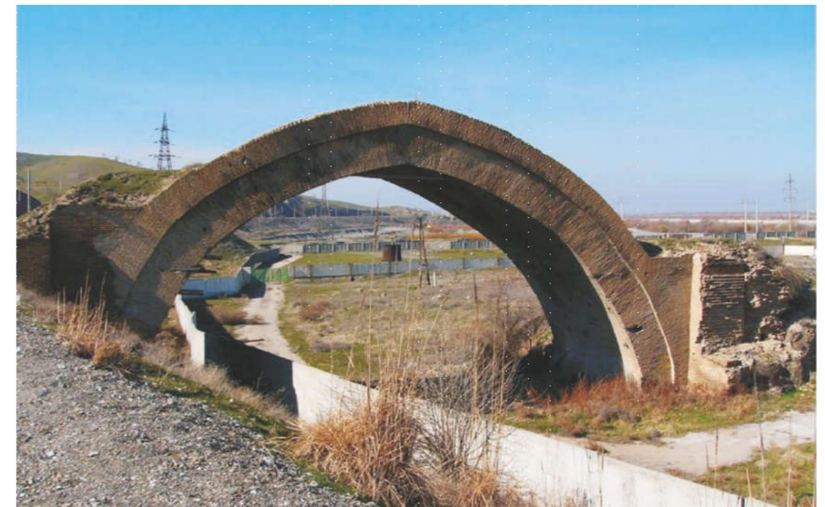
Figure 3. Remnants of the Ancient Bridge – Water Divider in the Zarafshan Valley (Shodman Malik, the 16th Century AD)
