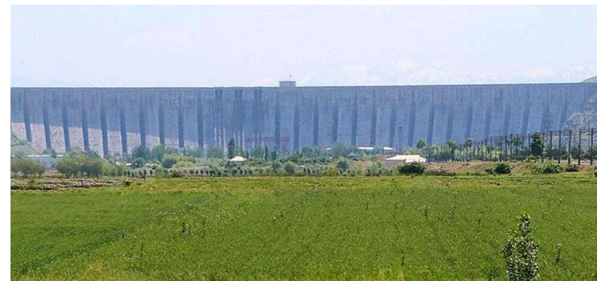
Figure 9. “Kampirravot” dam built on the Karadarya river. It was designed in 1962 and was completed in 1968-1982. The total length 1020 m. Dam is massive concrete with double buttresses-875 m. Maximum height 115 m.
