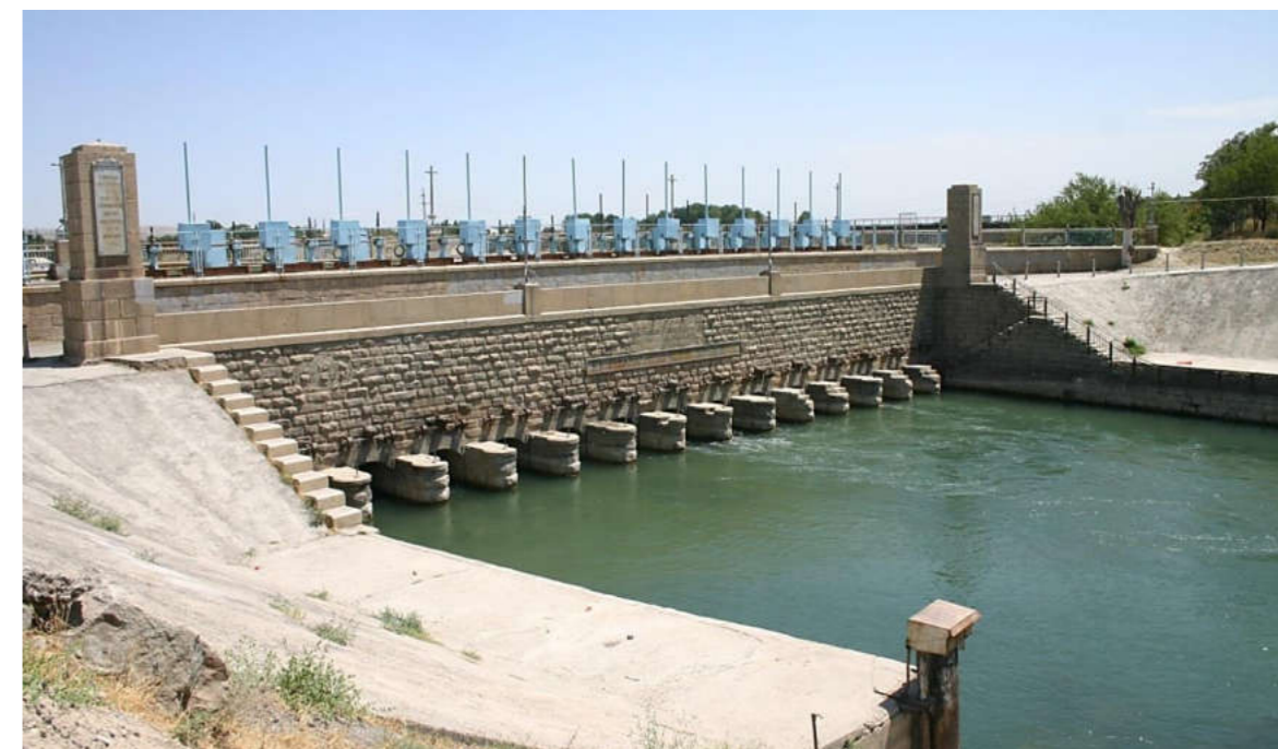
Figure 4. The head structure at the Dustlik (“Friendship”) canal (in the Soviet years, the Kirov Canal. It starts from the derivation channel of the Farhad hydroelectric station. Construction began in 1907 and was completed in 1913)
